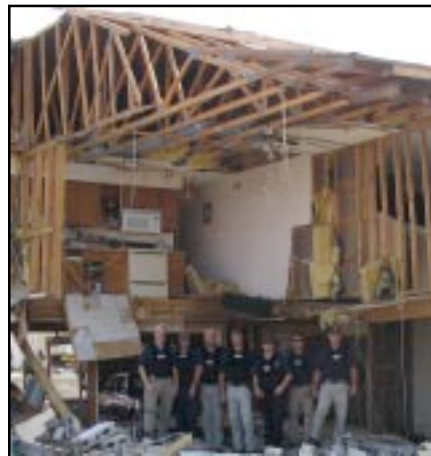
A quick response team inspects damage. NOAA
